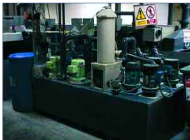
Copper Etchant Phase 1 Regeneration Chamber
